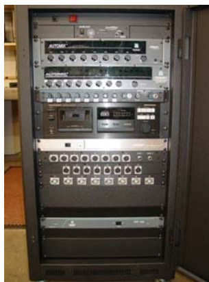
Another completed cabinet.
