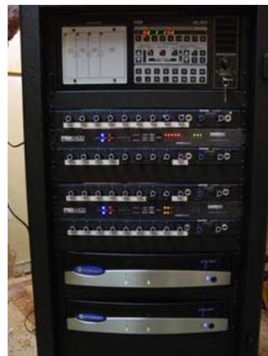
An operating cabinet.
