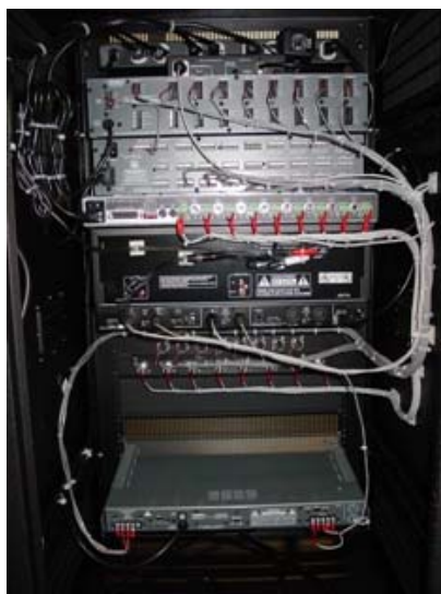
Structured wiring inside a cabinet.
